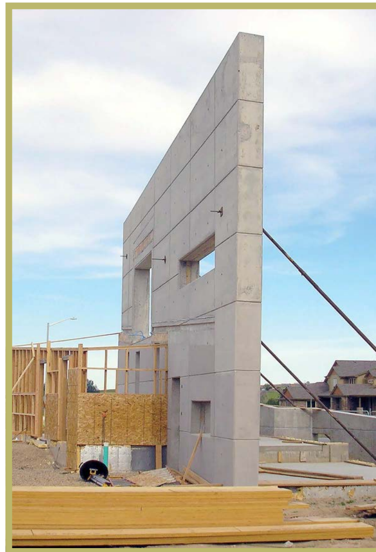
A central mass wall forms the spine of the home and also serves as a passive solar collector, radiating heat when interior temperatures drop.
